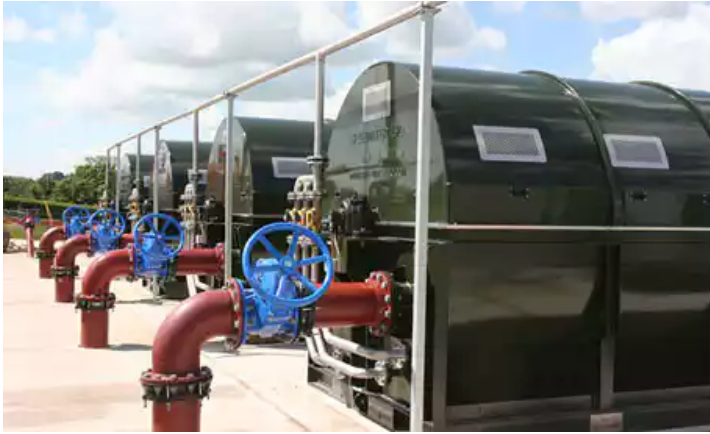
HYBACS Units at Ashbourne Sewage Treatment Works. The HYBACS system is a green more efficient way to deal with sewage. Photograph: Bluewater Bio
