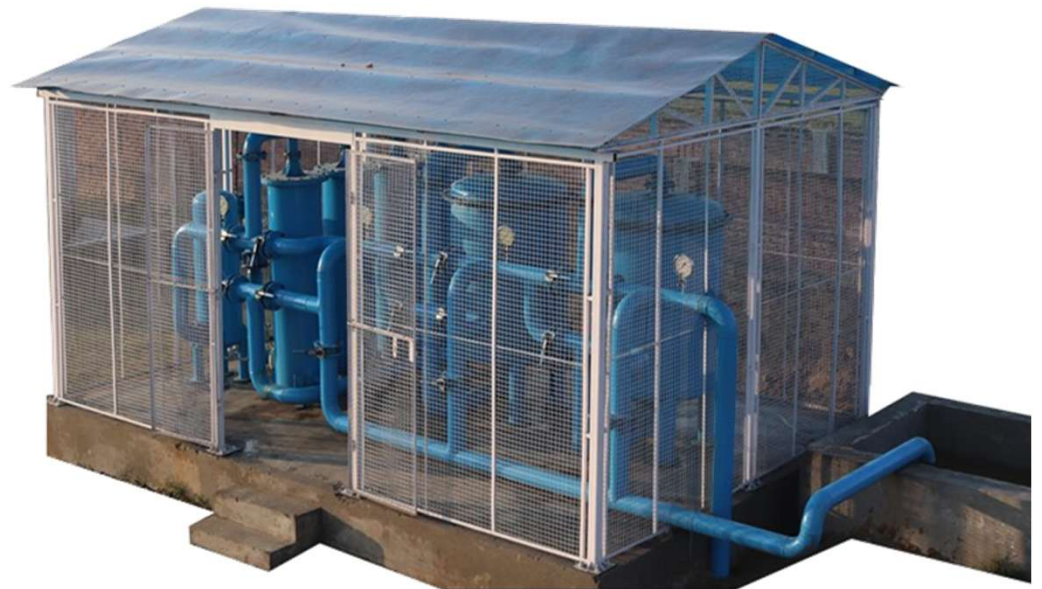
Retrofitted Water Purification Plant Capacity: 0.1-1 MLD
